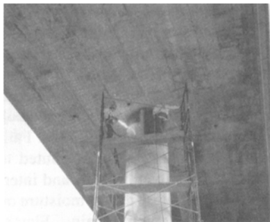
Application of powder coatings (Photos courtesy of Plastic Flamecoat Systems and CALTRANS)
