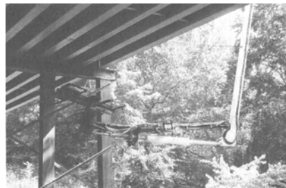
Video-equipped robotic platform moves toward corroded area during field test (Photos courtesy of North Carolina State University)
